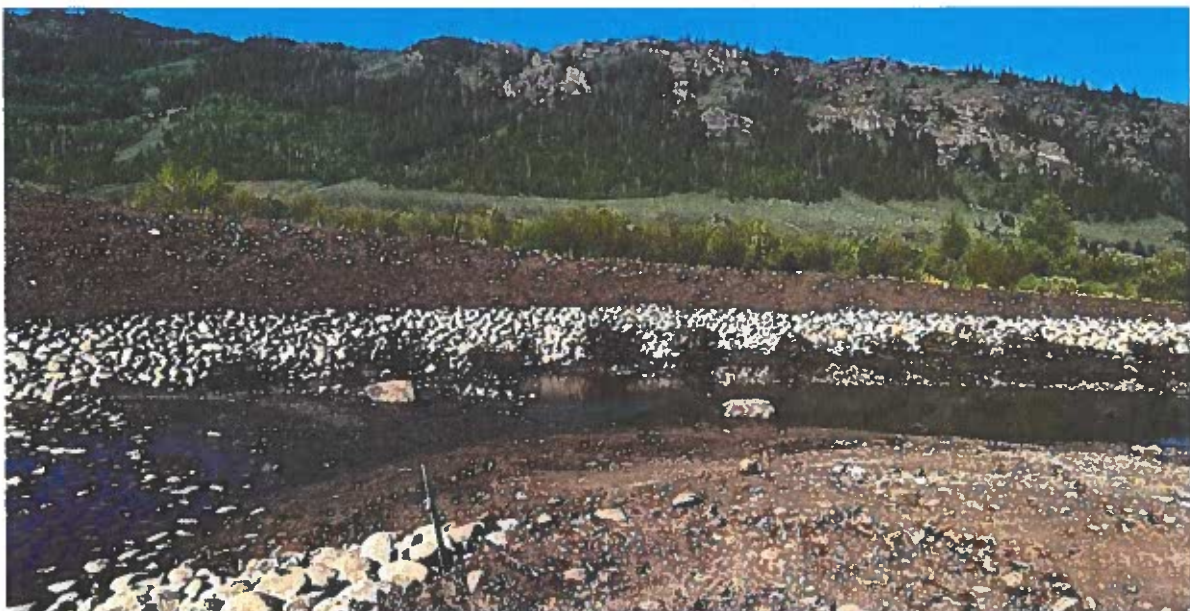
The Colorado River Connectivity Channel will connect two segments of the Colorado River near Windy Gap Reservoir.
