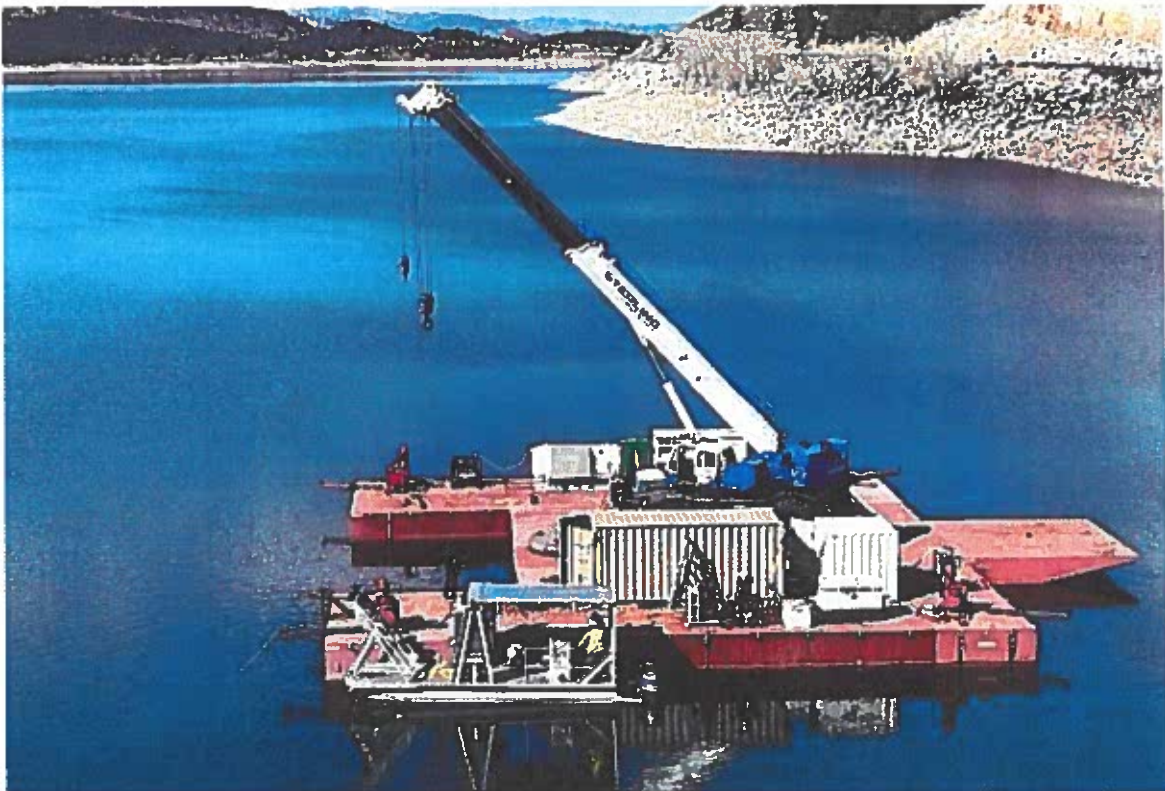
Crews work to install a bulkhead at Carter Lake before an inspection.
