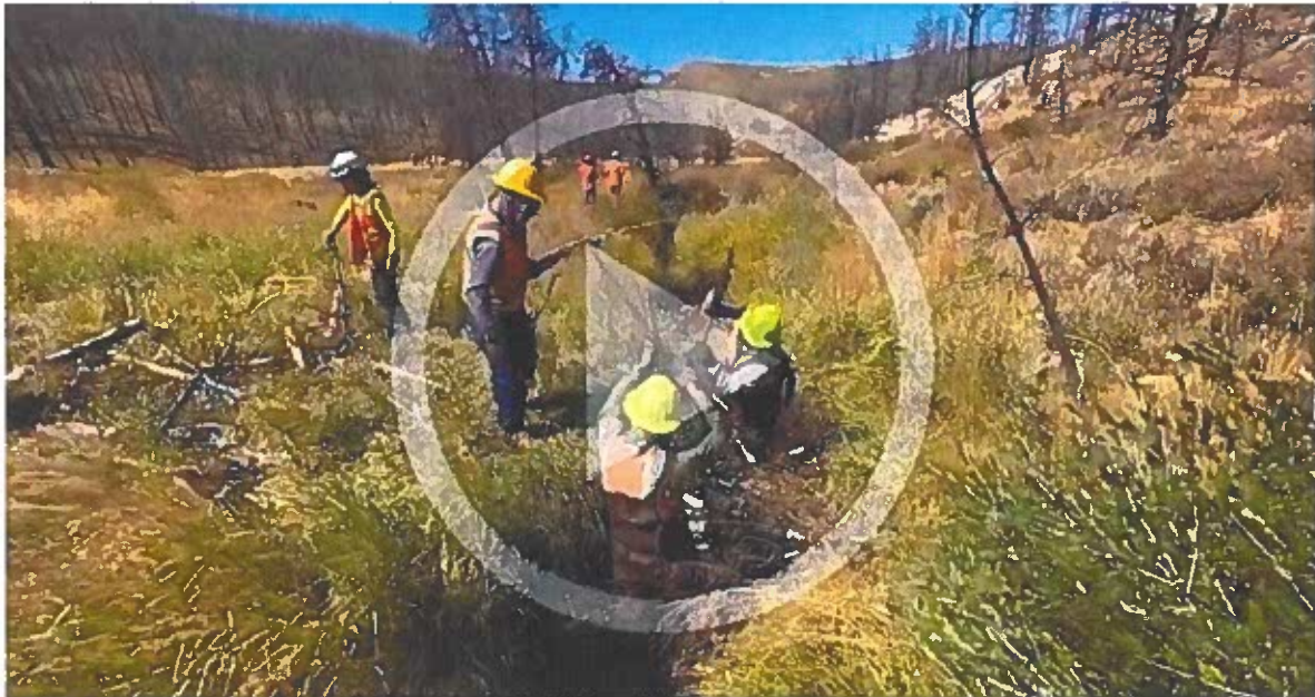
A crew works this fall to install post-assisted log structures in an area burned by the 2020 East Troublesome Fire.
