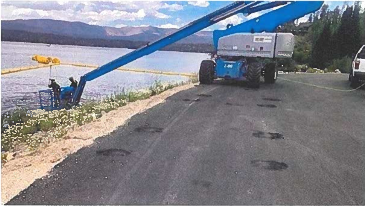
Northern Water Collections Systems Department workers use a boom lift to clear debris from the West Portal of the Adams Tunnel.
