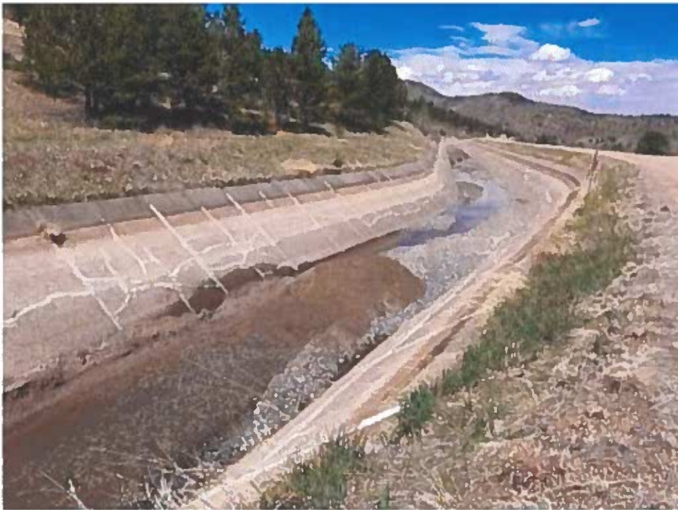
Sediment sits at the bottom of the Hansen Feeder Canal this spring. Crews removed nearly 1,000 tons of material that had entered the canal.
